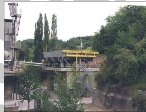
Industrial Waste Heat Recovery
