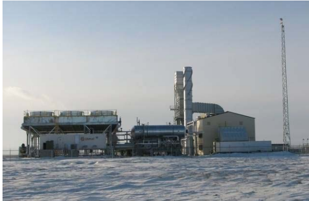
5.5 MW Kerrobert REG Project, Saskatchewan, Canada
