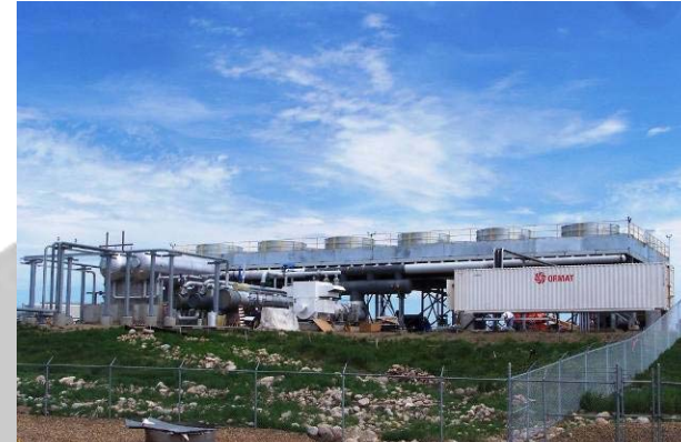
5.5 MW Northern Border Pipeline REG Project (OREG1), North Dakota
