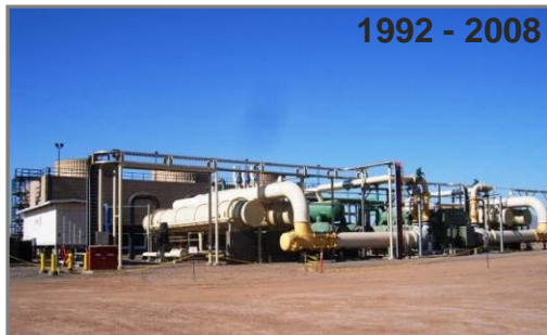
92 MW Heber Binary Geothermal Complex, California
