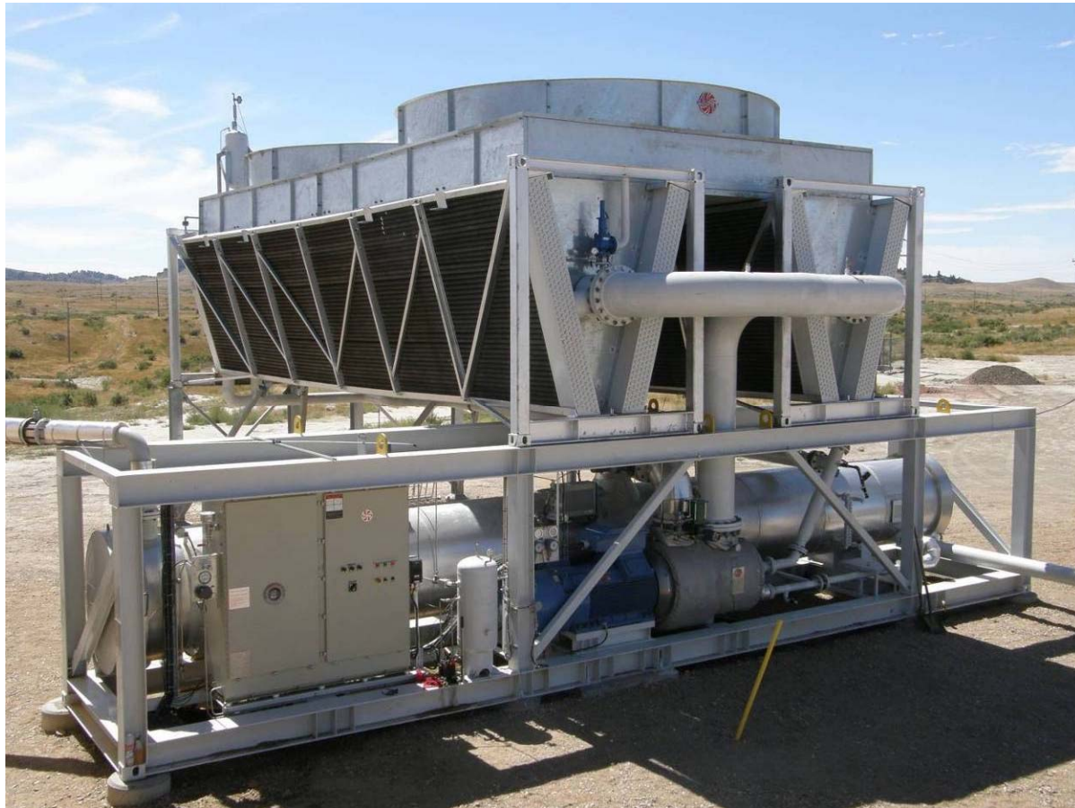
Rocky Mountain Oilfield Testing Center (RMOTC) being used for Ormat demonstration power plant
