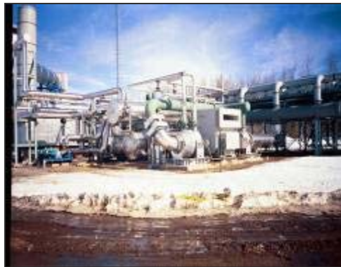
Heat Recovery - Pipelines
