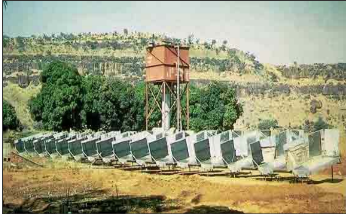
Solar Powered ORC Water Pump – Mali 1966
