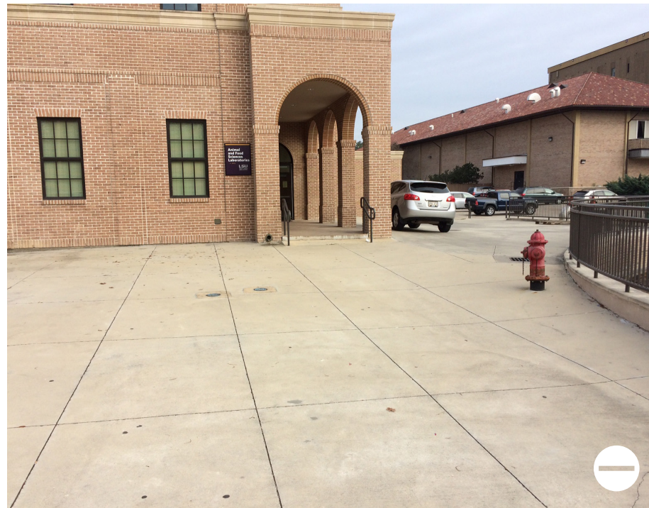
An insensitive linkage dominated by unarticulated concrete hardscape and lacking any landscape elements
