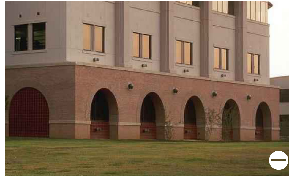
The Louisiana Emerging Technology Center replicates the arched form of the historic core's arcades, but blocks them in, removing their functionality as an inhabitable, connective space. The absence of landscaping and tree canopies creates a harsh pedestrian environment, as compared with the more human-scaled and layered building edges of the central core.
